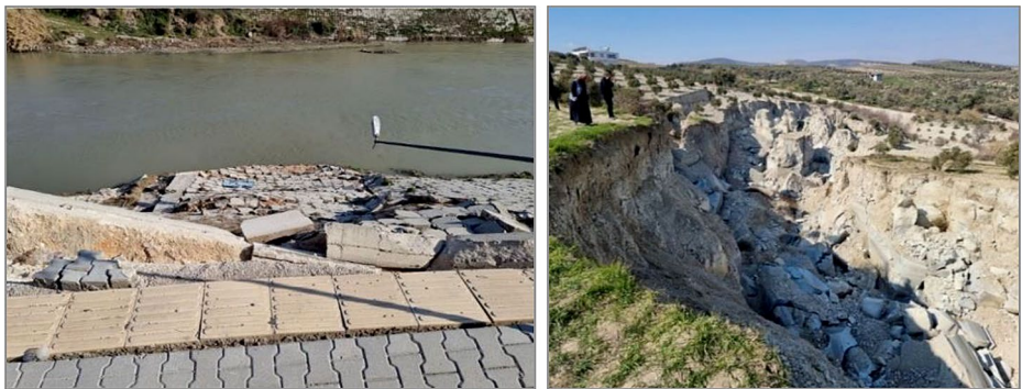
Fig. 7 Landslide damage observed in Antakya (left) and in Altınözü (right) districts of Hatay
