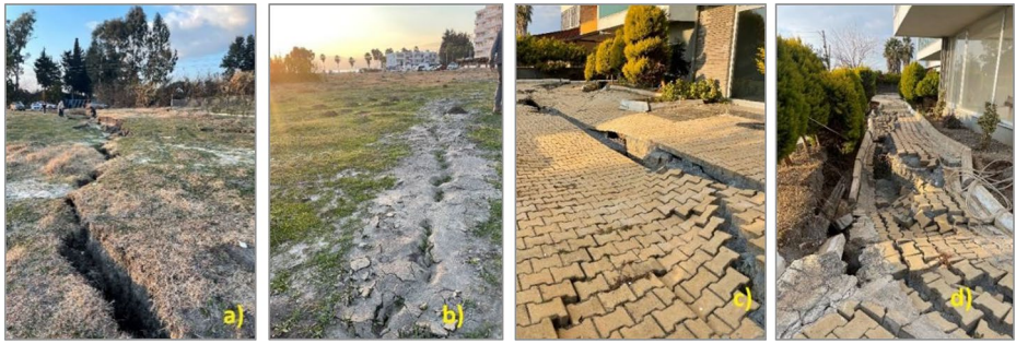
Fig. 6 Liquefaction-induced failures observed in Dörtyol district of Hatay
