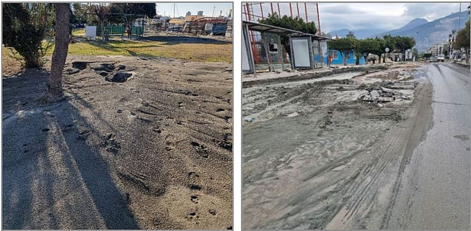
Fig. 5 Sand cones and crater geometries along the coastline (left) and some of the damages on road structures (right) in Iskenderun district of Hatay
