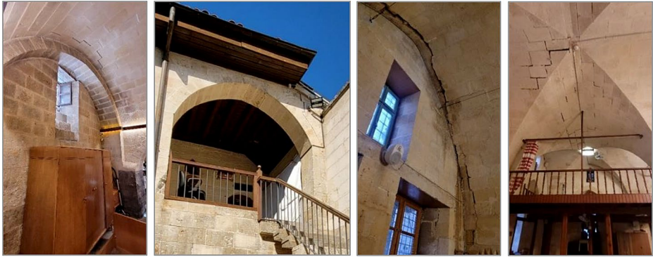
Fig. 26 Examples of tensile cracks at joints in arches, vaults, and domes, out-of-plane movements
