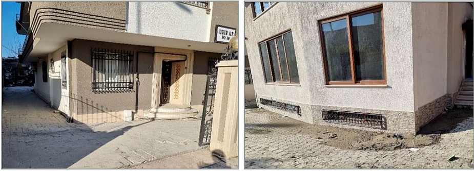
Fig. 4 Uniform settlement of a building (left) and sand ejecta around a structure (right) in Iskenderun coastal region of Hatay
