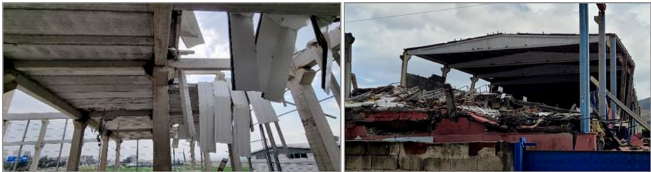
Fig. 19 Floor damage due to poor connection detailing (left) and a precast concrete structure with weak columns and heavy roof beams (right)
