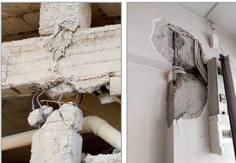
Fig. 14 Examples of a strong beam weak column design and damage on columns
