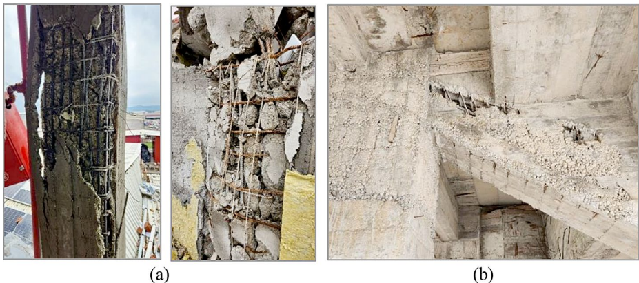
Fig. 10 Examples of poor concrete quality (a) and wrong placement of concrete (segregation) (b)
