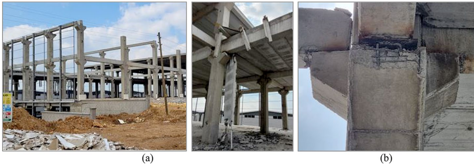
Fig. 18 Examples of insufficient fastening of roof purlins to beams (a), and damage in joint regions (b)
