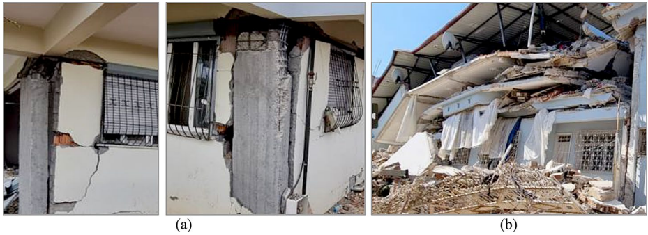
Fig. 16 Examples of column damage due to large overhangs (a) and a building collapse due to additional floors (b)
