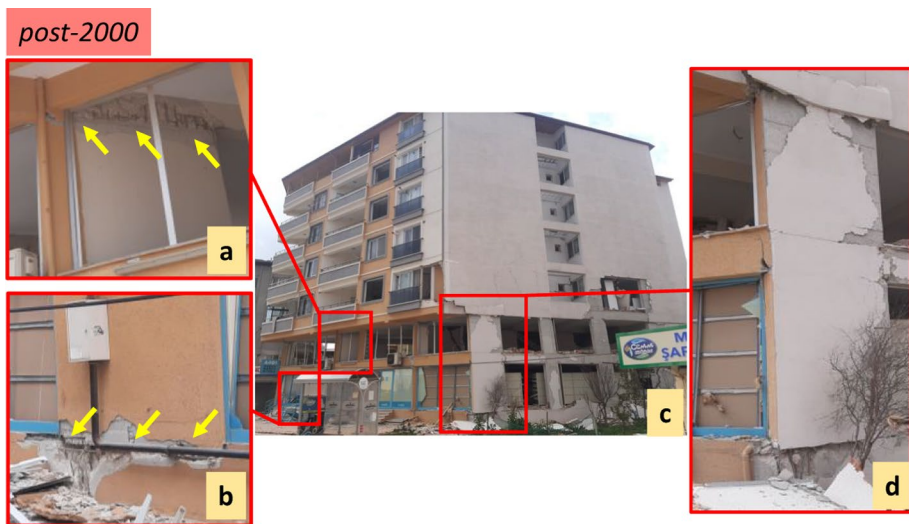
Fig. 21 In-plane sliding shear behavior between two adjacent wall segments (a) and out-of-plane sliding shear failure at wall-foundation interface (b–d) of a 7-story building (c) in Hatay
