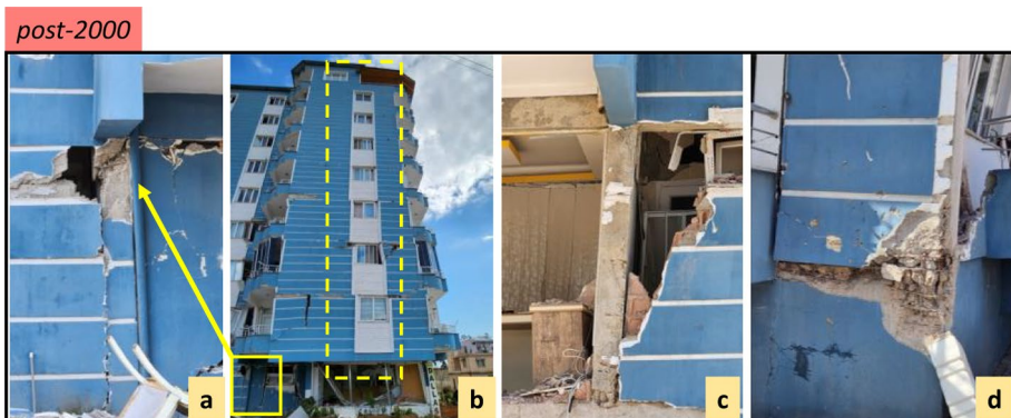
Fig. 24 Heavily damaged 10-story building in Hassa, Hatay with a large residual drift at first four stories (b), and out-of-plane bending and shear failure of the structural wall (a, c and d)
