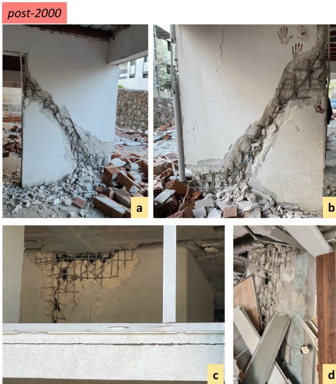
Fig. 19. 9-storey building with heavy damage in Hatay, presenting shear failure at both sides of a structural wall (a and b), 8-storey building with heavy damage in Hatay, with shear failure of structural walls (c and d)
