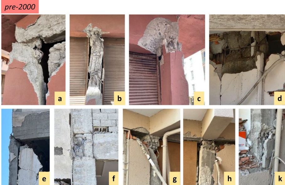
Fig. 17 Heavily-damaged building in Osmaniye, buckling of smooth reinforcement, shear failure of column & beam-column joint (a, b and c), Heavily-damaged building in İskenderun, pipeline passing through a column (d), shear failure of column & beam-column joint (e and f), Heavily-damaged building in Hatay, buckling of column reinforcement (g, h and k)
