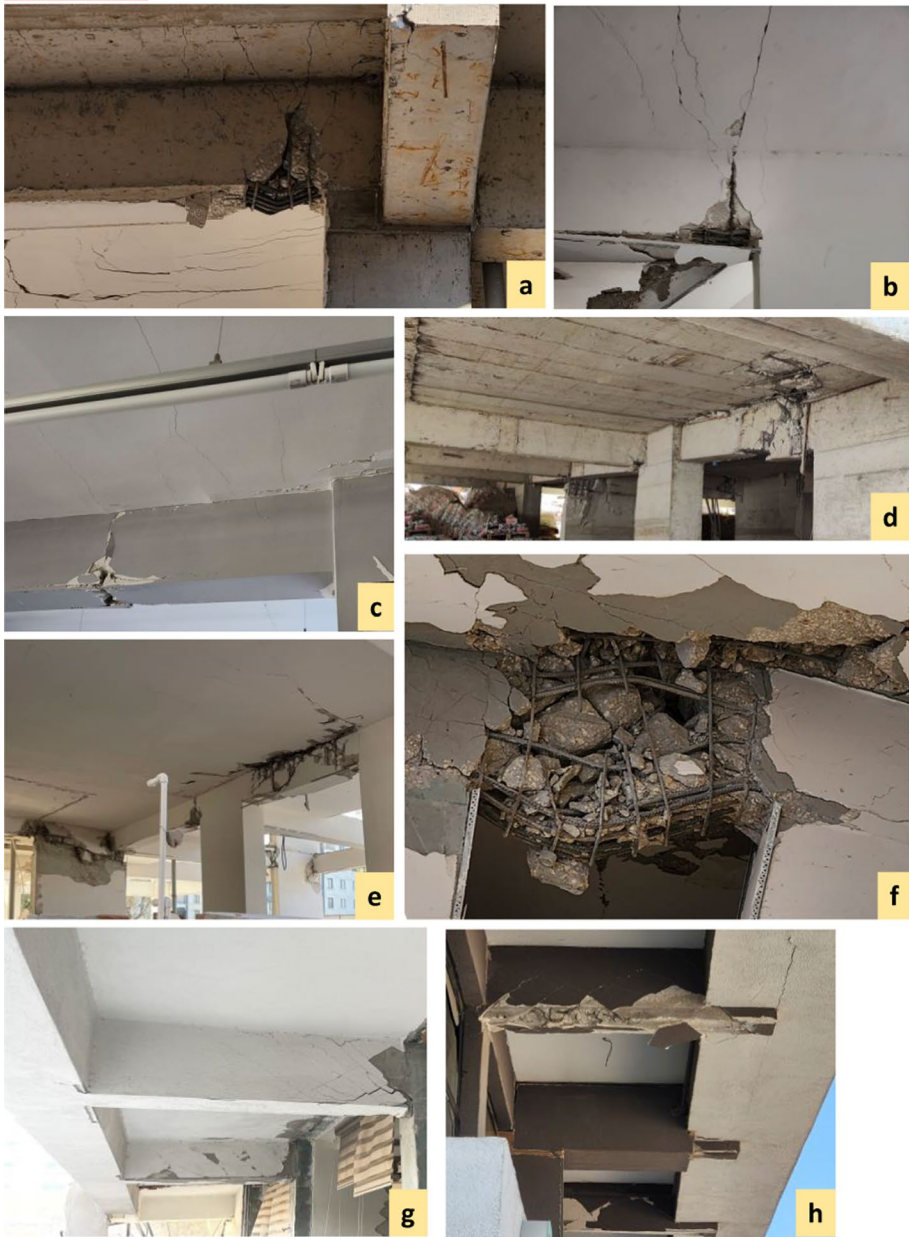
Fig. 25 Bending failure at the beam end zone (a), tension cracks at the beam support continuing through the slab (b), tensile crack at the one quarter of the beam span (c), and shear failures at relatively short beams of Altunpark 2 Sitesi Block C (d, e) in Hatay, shear failure of a coupling beam from a partially collapsed building in Hatay (f), cantilever beam failures (g, h)
