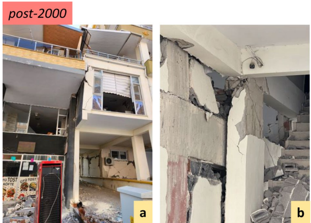
Fig. 16 Hammering of two adjacent buildings in Hassa, Hatay (a), inside look from the building on the right (b)
