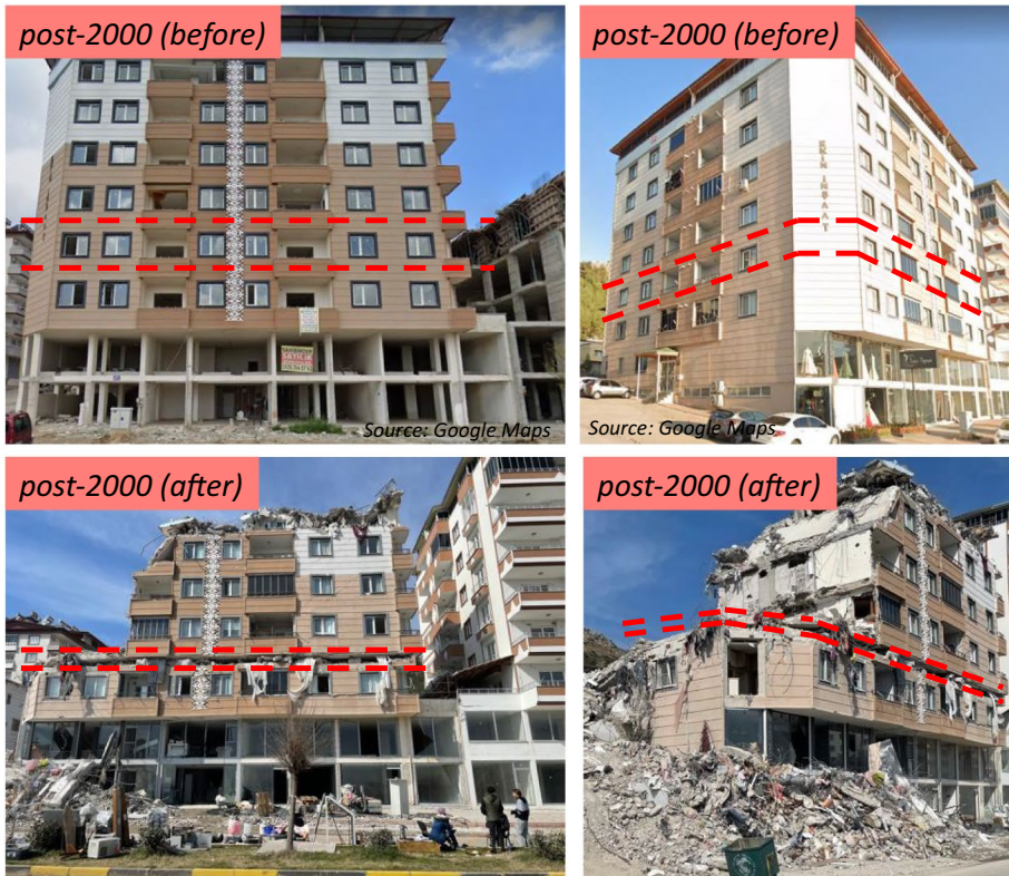
Fig. 9 Collapse of the intermediate story of a post-2000 building in İslahiye (note that the left side of the building was being demolished at the time of the reconnaissance visit)
