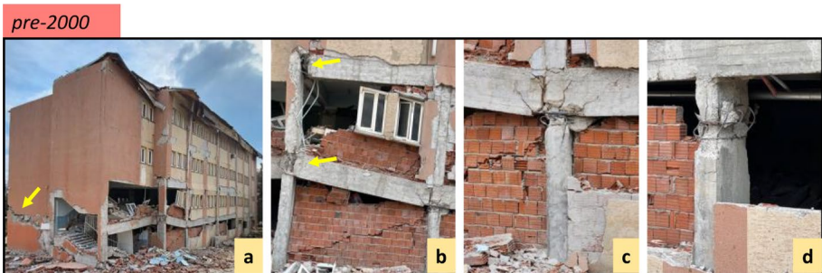
Fig. 18 Old school building with heavy damage in Nurdağı, Gaziantep, shear failure of the shear wall (a), shear failure of beam-column joints (b), and buckling of column reinforcement (c and d)
