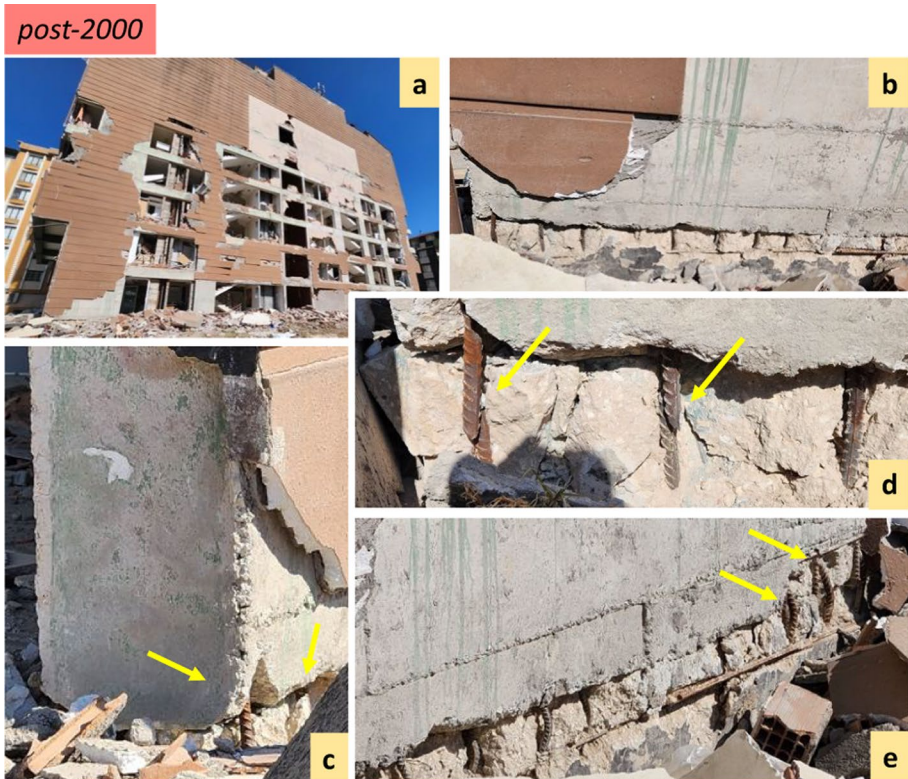
Fig. 23 Heavily damaged building in Hatay (a) with out-of-plane shear failure of RC wall, resulting in brittle shear failure, fracture and buckling of the vertical reinforcement (b–e)
