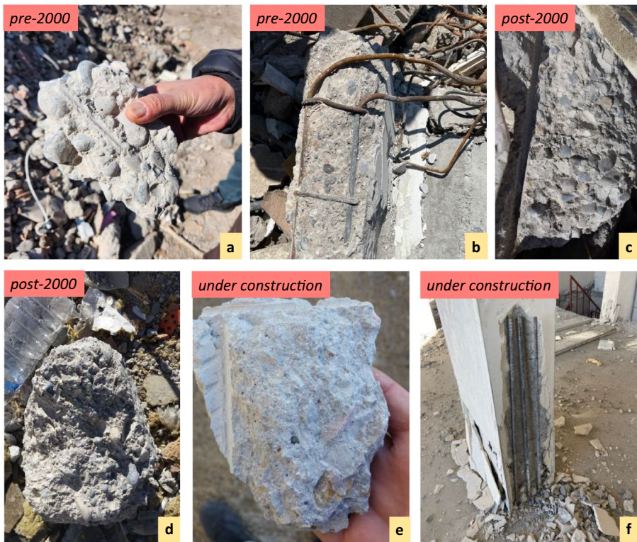
Fig. 4 Partially collapsed pre-2000 building in Osmaniye with inappropriate aggregate and mixture of concrete (a), bond failure of corroded smooth reinforcement (b). Heavily damaged post-2000 building in Kahramanmaraş with inappropriate aggregate and mixture of concrete (c and d). Heavily damaged under construction building in Malatya with inappropriate aggregate and mixture of concrete (e) and lap splice of reinforcement (f)
