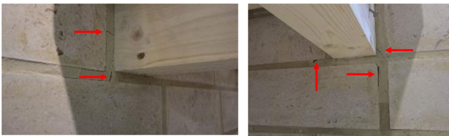
Fig. 14 Mortar cracks due to shrinkage near a timber beam
