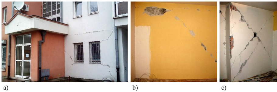
Fig. 30 Performance of type M3-M multi-family residential buildings in the 2010 Kraljevo, Serbia earthquake: a diagonal and horizontal cracks in an exterior wall; b in-plane damage of a load-bearing interior wall (solid clay bricks), and c extensive cracking in a partition wall (multi-perforated clay blocks) (Blagojević 2022)
