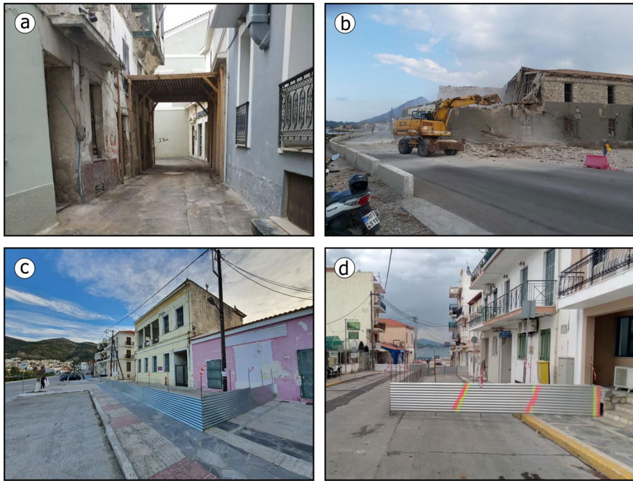
Fig. 7 Actions for the mitigation of hazards in the aftermath of the earthquake in Samos island: a supporting of buildings, b demolition of unstable buildings dangerous for cars and passersby, c , d placement of markings and protective barriers around severely affected buildings in order to avoid approaching
