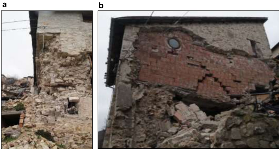
Fig. 23 a Project 8 (Campi Alto): crumble of masonry walls at ground floor; b Project 2: collapse of the masonry walls at ground and first floor
