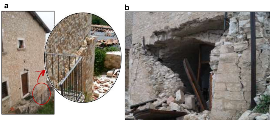
Fig. 22 Project 4 (Campi Alto): a rigid rotation of replaced floors with respect to the ground floor; b crumble and collapse of poor masonry wall at ground floor
