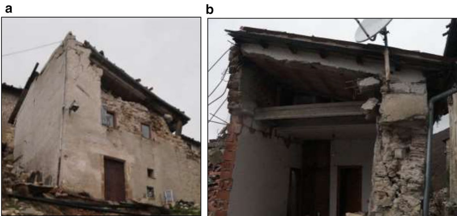
Fig. 24 Project 11 (Campi Alto): collapse of poor quality masonry walls due to the presence of heavy roof: a downstream façade; b lateral section
