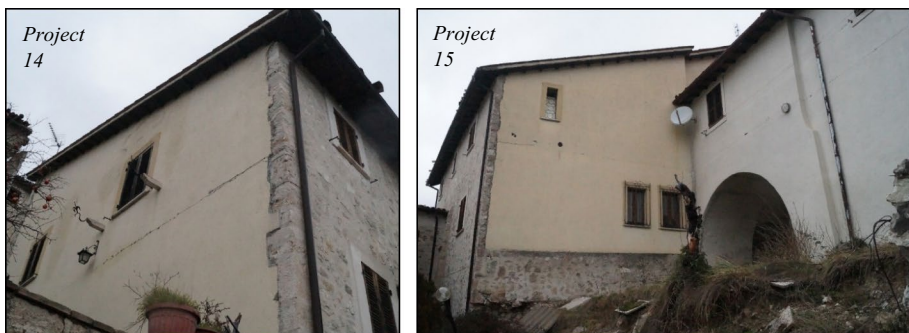
Fig. 19 Common horizontal cracks at floor level of MSUs located in Campi Alto
