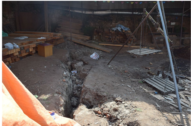
Fig. 4 Liquefaction and cracks in the ground at Kausaltar, Bhaktapur, Nepal, after the 2015 Gorkha earthquake, (Location 7a on Fig. 2). Photograph taken on 2015-05-31 [RM Pokhrel]
