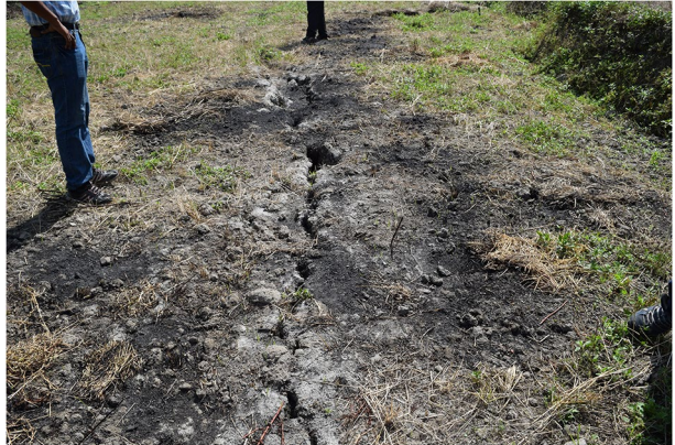
Fig. 10 Liquefaction and sand boiling at Bungmati (Liq. ID 3a in Table 6) [Photo: RM Pokhrel]
