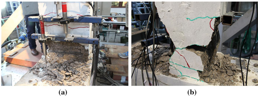
Fig. 8 Structural damage in FF-WC and FF-LC columns at 500% excitation (complete damage): a FF-WC and b FF-LC
