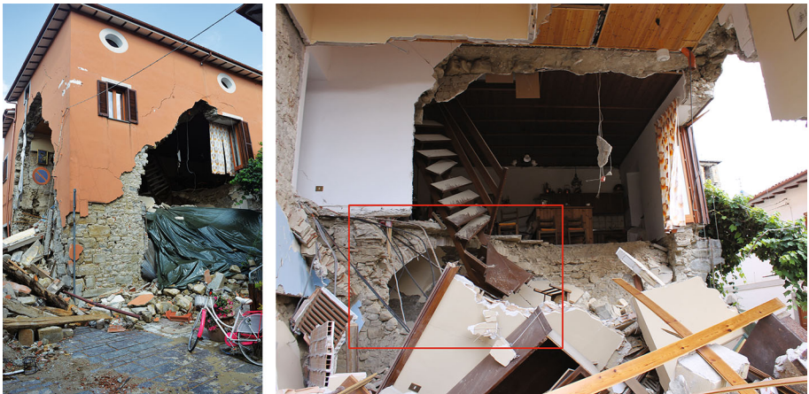
Fig. 24 Residential masonry building: D5 damage level
