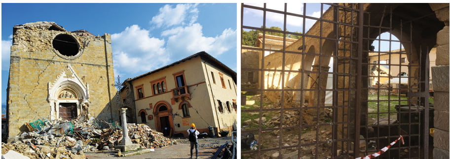
Fig. 26 Church of S. Francesco: damage level D4, collapse of tympanum (M6) and in-plane cracking of façade (left); collapse of columnnade (right), ev1 vulnerability factor
