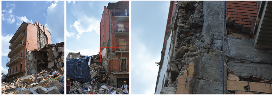
Fig. 27 Residential RC building (damage level D3): global damage (left), damage of beam-column node (center), particular of the node (right). Damage mechanism MC, vulnerability factor e_vD
