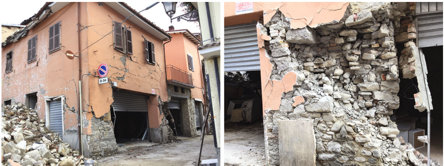
Fig. 23 Residential masonry building: D4 damage level, shear failure of external walls mechanism (M1), poor masonry vulnerability factor (ev4)
