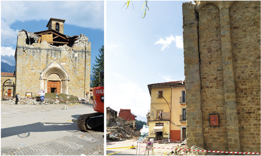
Fig. 25 Church of S. Agostino: damage level D4, collapse of tympanum (M6) and in-plane cracking of façade (left); overturning of façade (M3, right), ev1 vulnerability factor
