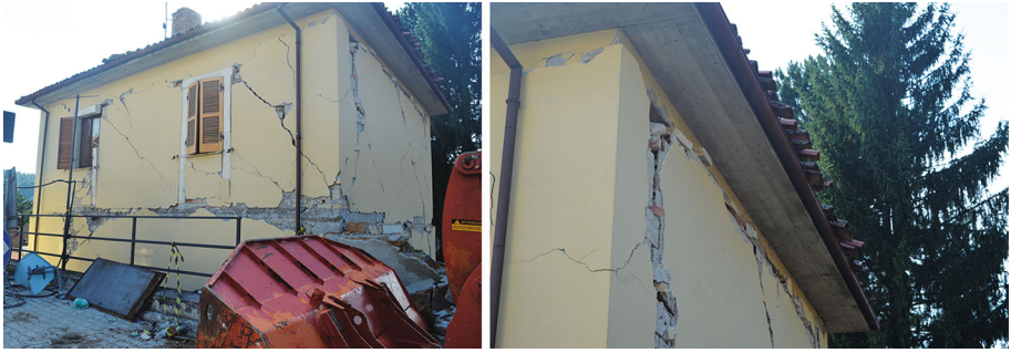
Fig. 22 Residential masonry building: D3 damage level, in-plane cracking shear mechanism (M2), poor masonry vulnerability factor (ev4)
