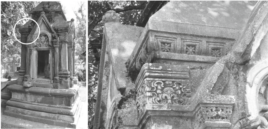
Fig. 8 Earthquake damage to the Payar temple has occurred through lateral displacement of the monolithic roof capstone. At some time in the past nine centuries the roof capstone has shifted \approx 7 cm northward, with no damage to the underlying dressed stone blocks. We attribute the drift of the roof monolith to shaking during earthquakes. A close-up of the offset NW corner of the shifted roof stone is shown right, which, in our opinion, Kak (1933) erroneously diagnoses as a failed attempt to dismantle the temple
