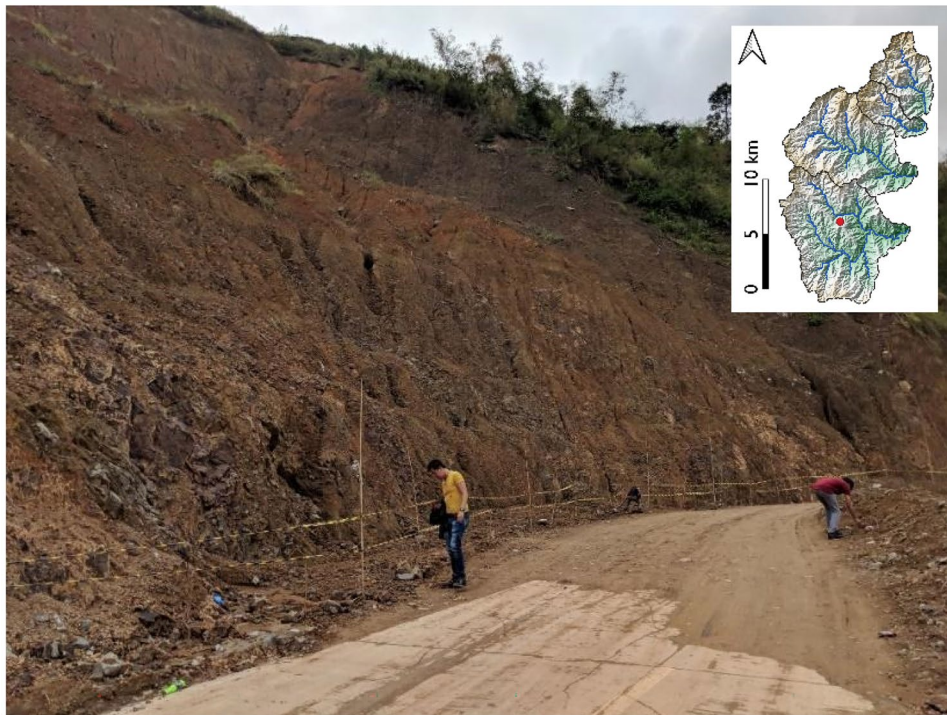
Fig. 4 View of the slope that was affected by one of the major landslides during Typhoon Mangkhut (2018). Inset, the red dot shows the location of the picture in the study area. Photo credit G. Bennett
