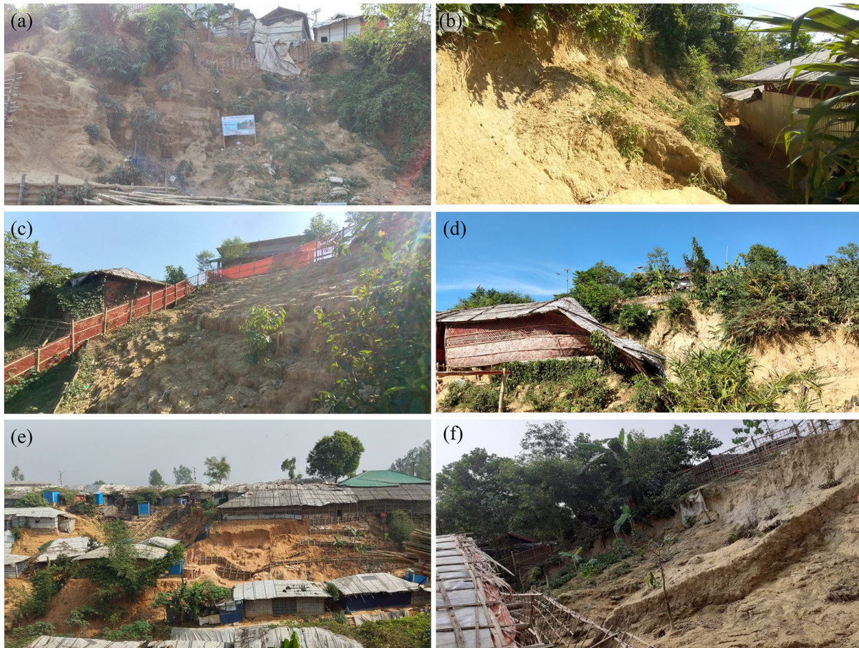
Fig. 3 Landslides in the Kutupalong Rohingya Camp (photos taken during the fieldwork). a Camp 18 (slump). b Camp 4 (rotational slide). c Camp 20 (creep with polygonal tension cracks). d Camp 17 (slump/debris flow). e Camp 8E (slump). f Camp 5 (rotational slide)
