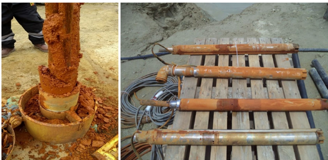
Fig. 13 Examples of accumulation of oxides in pumping equipment (courtesy Julio Larota)
