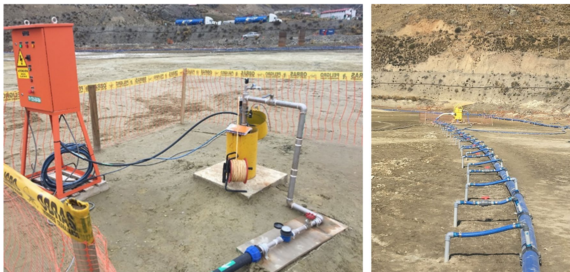
Fig. 6 A pumping well (left) and a wellpoint line (right) in the B2 TSF (Courtesy Julio Larota)
