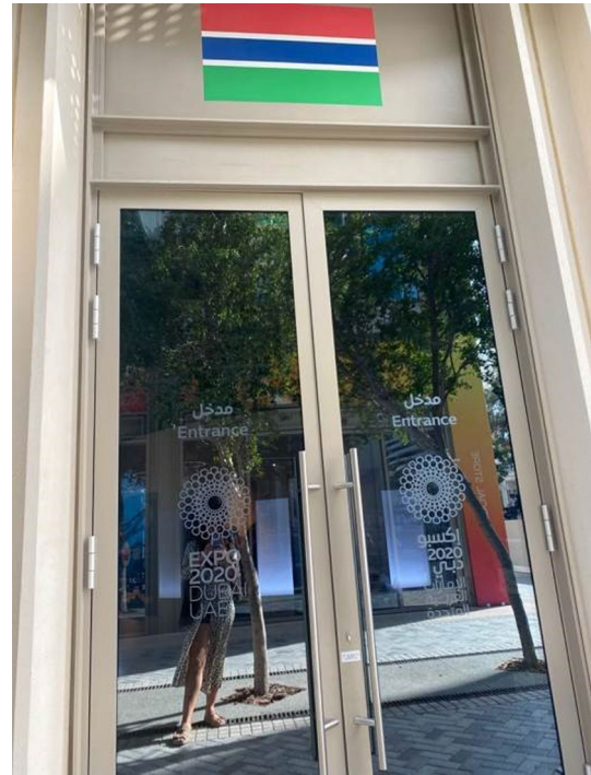
Fig. 10 Manual doors in small pavilions
