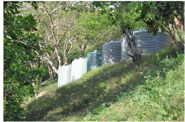
Fig. 2 The five water tanks waiting to be connected to the the village infrastructure
