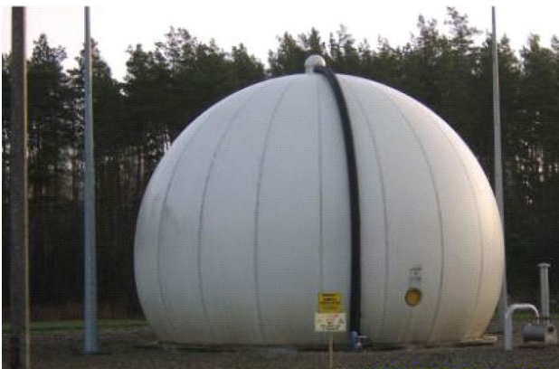
Fig. 2 Installation for the energy use of biogas from a sewage treatment plant in Nowa Wieś Elcka (Igliński et al. 2020b)
