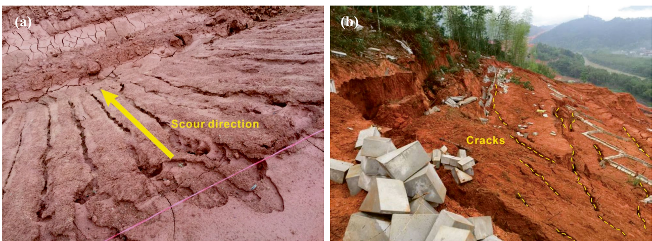
Fig. 7 Deformation and sliding of the fourth slope: a rain erosion (March 2016) and b cracks at the slope crest (April 2016)
