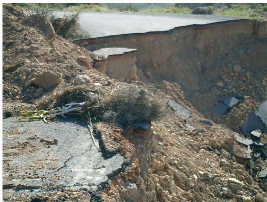
Fig. 4 The crest of the eastern sliding “slide 2”
