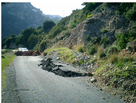
Fig. 5 The toe of the western sliding “slide 1”
