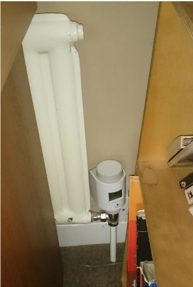
Fig. 1 Providing access to inaccessible controls
