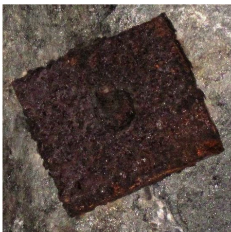
Fig. 4 Fully grouted uncoated rebar with unprotected steel accessories in the Hamregjøel tunnel after 47 years in service (Ongstad 2012)
