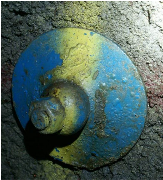
Fig. 12 Blisters observed in the rock bolt plate in the Oslofjord sub-sea road tunnel after 10 years of exposure (Ongstad 2012)
