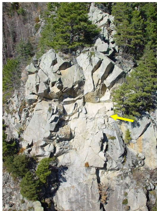
Fig. 2 Small rock bridge breakage (arrow) on the sliding plane
