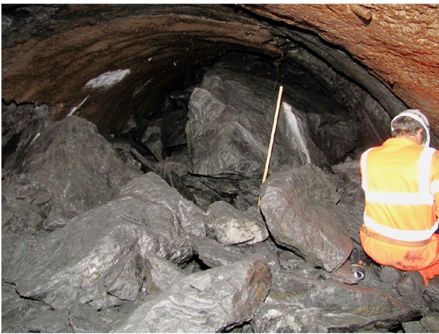
Fig. 12 Collapsed ground (downstream end). Note that the ground is largely made up of large fallen blocks (according to this photo). Photograph from Woolman (2016)
