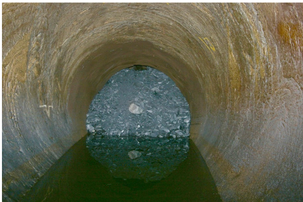
Fig. 10 Collapsed ground (upstream end)—taken from Woolman (2016). Note folded and faulted rock in the walls of the tunnel. This must be close to the fault zone. Note that the rock mass is broken down to very fine material, which is remarkable, given the decision not to line this section, and that no one could see the fault. The interpretation is that the material in situ was disintegrated, probably by tectonic action, rather like the ‘Rashings’ material in the South Wales Coalfield which looks intact but on extraction breaks down to sigmoidal fragments
