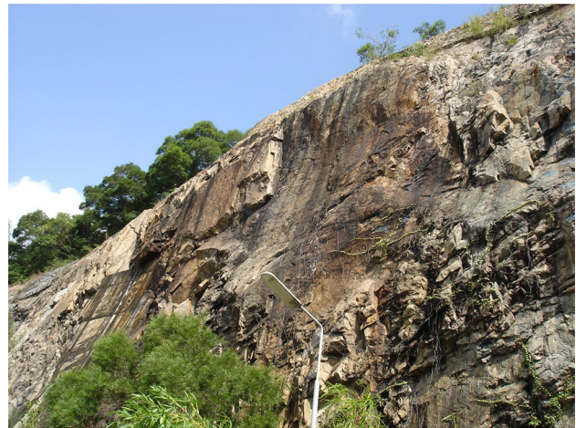
Fig. 5 Undercut blocks sitting on steeply dipping planes
