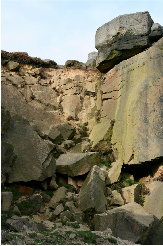
Fig. 3 Unexpected failure in the corner of the Cow and Calf Quarry
