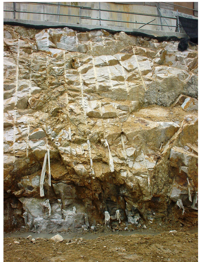
Fig. 3 Expansive chemical grout employed in pre-drilled holes to form rock cut slope. Castle Peak Road formation works, Hong Kong
