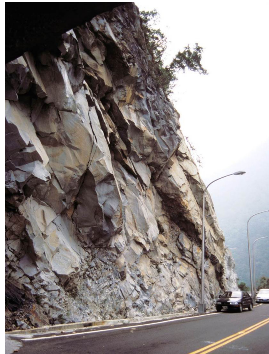
Fig. 1 Slope with daylighting rock slabs threatening highway in central Taiwan. The incipient nature of the discontinuities contributes tensile and shear strength and allows temporary stability
