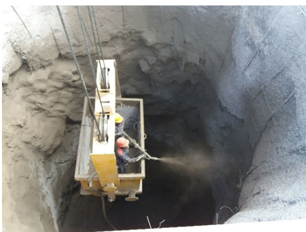
Fig. 4: The shaft excavated and supported for the assembly of the new cutterhead
