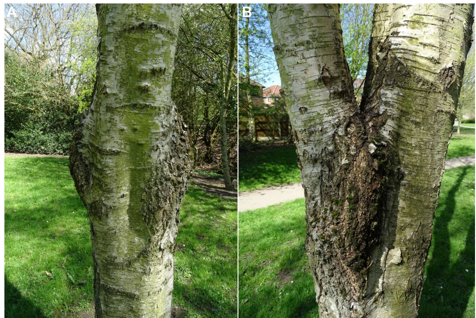
Fig. 1 A bark-included branch junction in silver birch ( Betula pendula Roth.) exhibiting considerable bulging at this bifurcation. a View of the bulging in-line with the bifurcation. b View of the bulging perpendicular to the bifurcation
