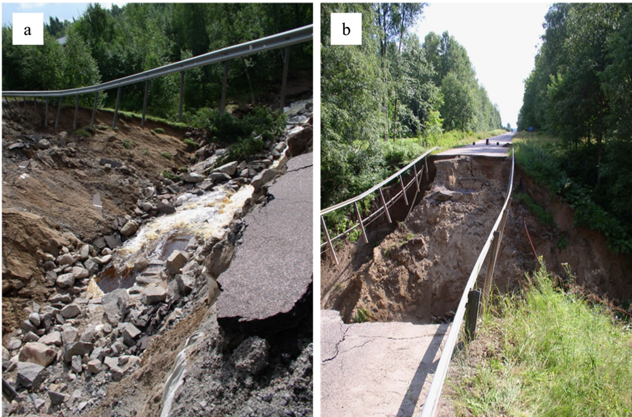
Fig. 3 a and b : Road and embankment failures in Värmland County 2004. With permission from Thomas Morling, Swedish Transport Administration
