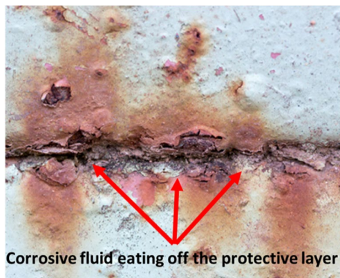
Fig. 7 Crevice corrosion on mild steel plate surface protected with paint [66]
