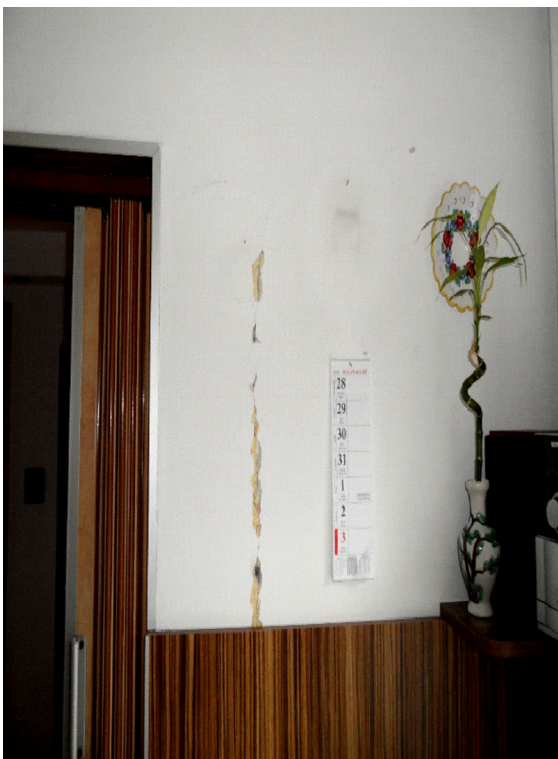
Figure 1 A vertical crack on a wall in the ground floor room
