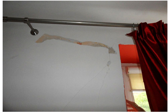
Figure 2 Cracks near the window
