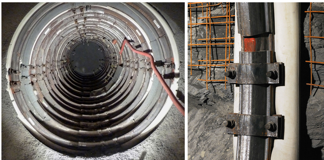
Fig. 4 The photo on the left shows the 12 m long shotcrete-free interjacent sealing section (ISS) at the end of the FE tunnel; the photo on the right shows a detail of a steel set bedded on a grout-injected hose for an even load distribution from the rock
