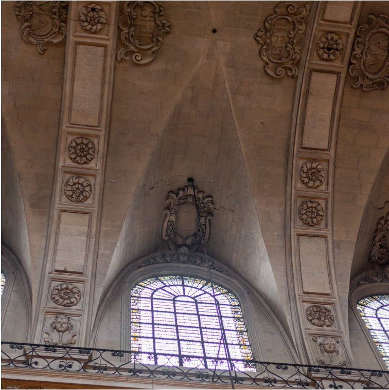
Fig. 13 Rectangular groin vaults in the Church of Saint-Paul Saint-Louis in Paris, built by François Derand. Image: author
