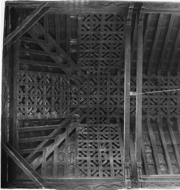
Fig. 1 Roof frame of the mosque in Marrakech (Morocco) (12th century). Photo courtesy of Christian Ewert
