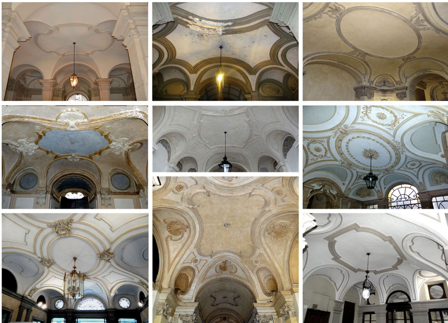
Fig. 2 Planterian vaults in the historic city centre of Turin, identified by their addresses: via della Consolata 12, via Corte d’Appello 13, Piazza Emanuele Filiberto 15, via Santa Chiara 8, via Botero 8, via Barbaroux 25, via Santa Teresa 1 g, via Santa Teresa 10, via Garibaldi 53. Photo: Author
