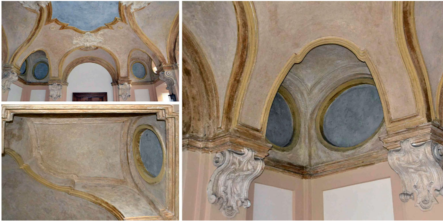
Fig. 13 via Santa Chiara 20 (Casa Martin Di Montù Beccaria): the model adheres to the architecture, albeit partially (adequately but with some deviation): the angular surfaces are realised by 'cuts and fills'
