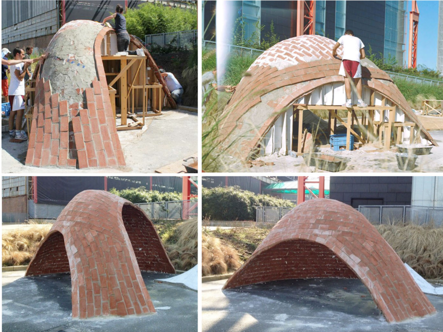
Fig. 20 The process of constructing the second layer of the Catalan vault according to the pre-modeled brick pattern
