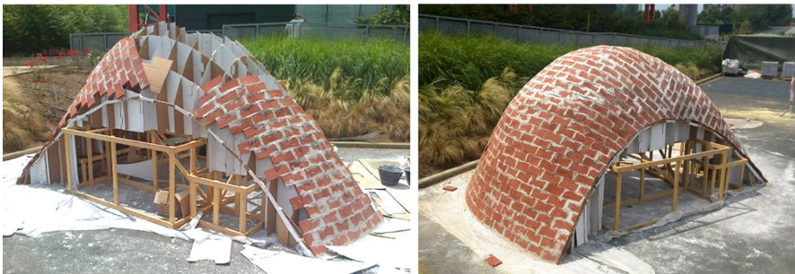
Fig. 19 The process of constructing the first layer of the Catalan vault according to the pre-modeled brick pattern
