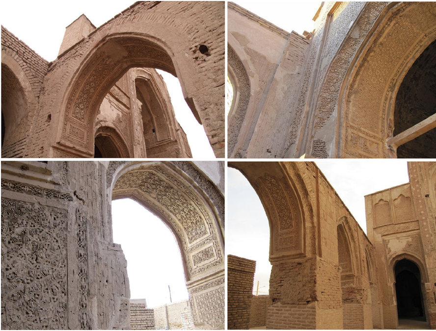
Fig. 4 Detailed view of the architectural ornaments located at the interior parts of the mosque
