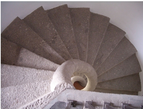
Fig. 2 Helical stair by radial solution. Colegio de Arzobispo Fonseca in Salamanca (Spain)
