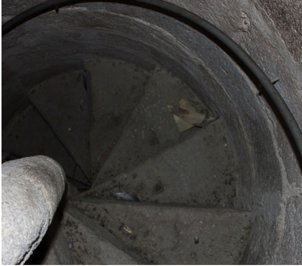
Fig. 6 Helical staircase by tangent solution. Church of Santiago Apóstol in Villa del Prado (Spain)
