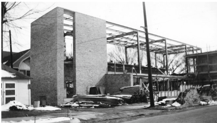
Fig. 12. Building construction, view of side aisle and sanctuary from street. Image © Christ Church Lutheran Archives
