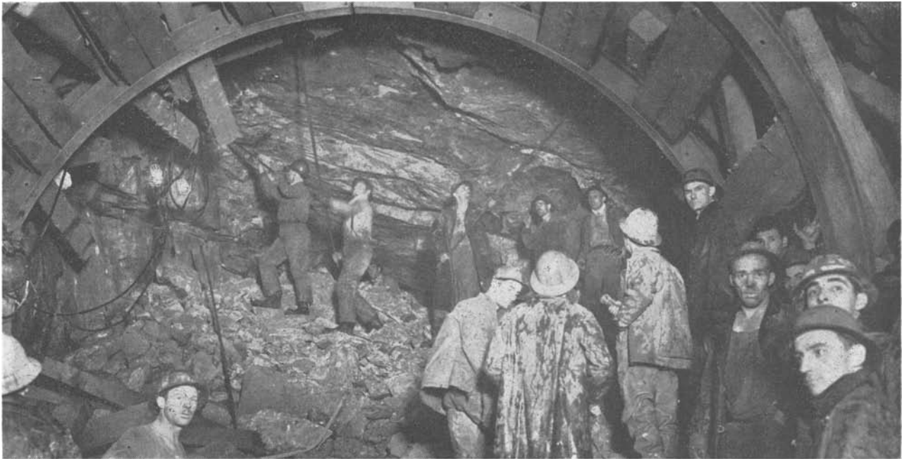
Barring down after the blast which holed through the San Jacinto tunnel. This tunnel pierced 13.04 miles of solid rock in the San Jacinto mountain range and was the most difficult unit of the entire metropolitan aqueduct construction.
