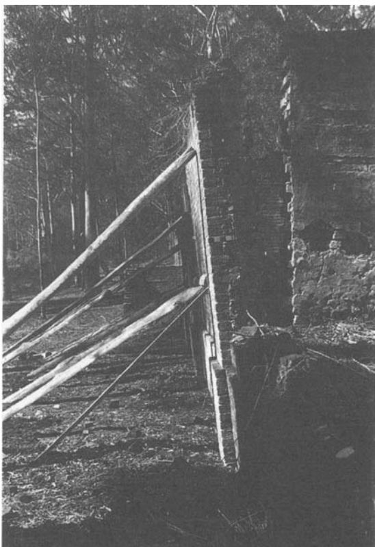
FIGURE 9. Leaning brickwork at the western end of the northern perimeter wall of the stables. The lack of foundations has brought this wall close to the point of collapse. Scale in 1 cm and 5 cm divisions. (Photograph by Bryan Asha, Kenthurst, NSW, 1993.)
