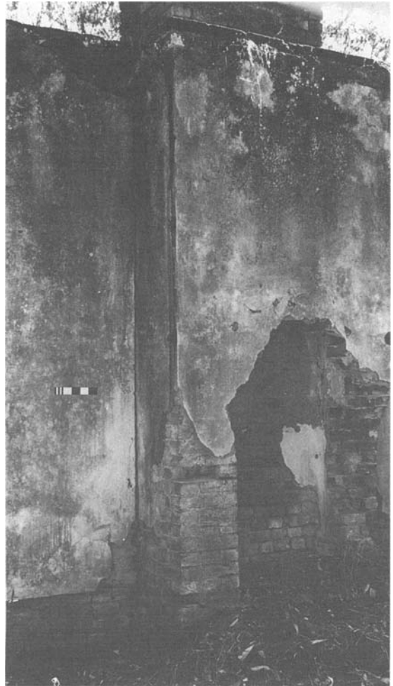
FIGURE 8. Bedroom fireplace in room at 14 in Figure 4. Note the lime-plastered walls, the header bond used at the back of the hearth, and the spaces left for wooden blocks to which the fireplace surround and the skirting board were attached (all the rooms in the house had suspended timber floors). Scale in 1 cm and 5 cm divisions. (Photograph by Bryan Asha, Kenthurst, NSW, 1993.)
