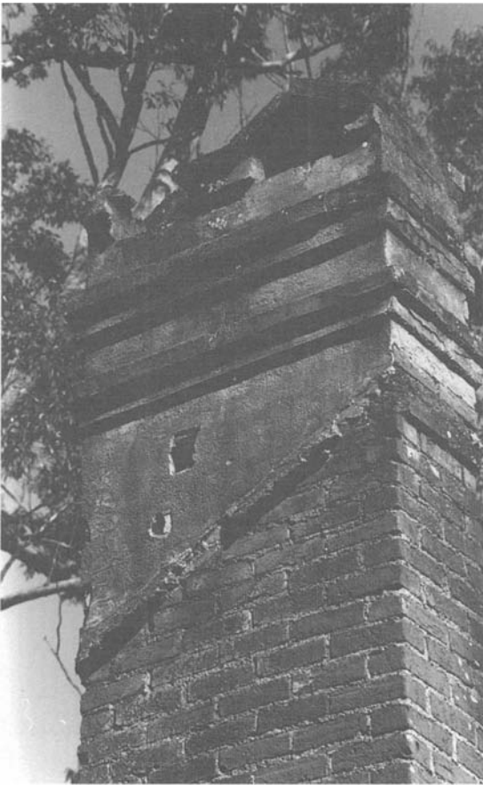
FIGURE 7. Eastern side of the bedroom chimney serving rooms at 9 and 10 in Figure 4. Note the scribed rendering over the stretcher-bond brickwork and the indications of a shingled, pitched roof. (Photograph by Bryan Asha, Kenthurst, NSW, 1993.)
