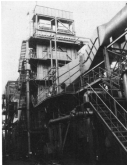
SINTERING PLANT off-gas desulfurizing unit recently installed at Kawasaki Steel Corp.'s Chiba Works can treat 120,000 normal cu meters of gas hourly.
