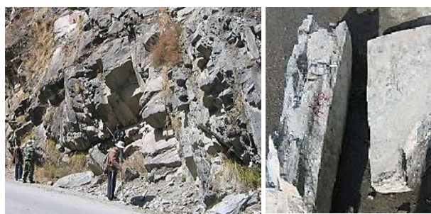
Fig. 4 Side and close-up view of rock slope showing fracturing and dimension of the rock mass
