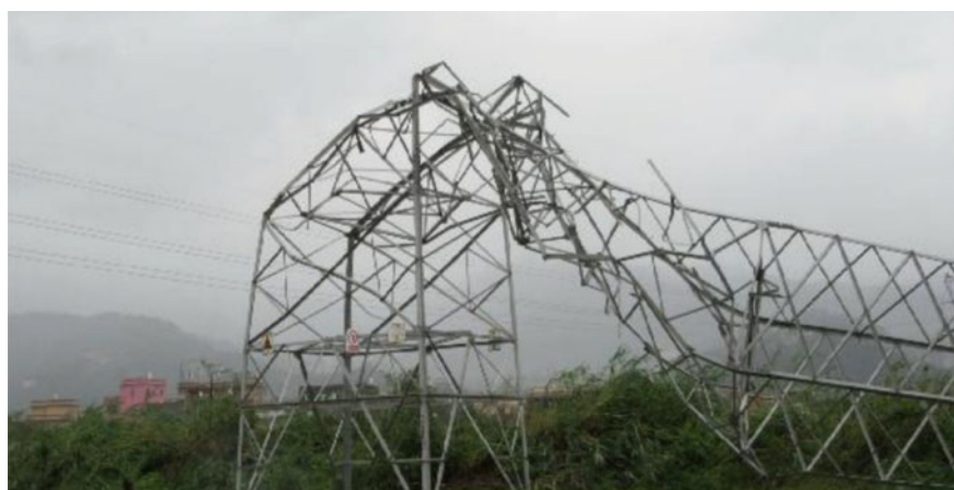
Fig. 3.12 Damage scene of power tower
