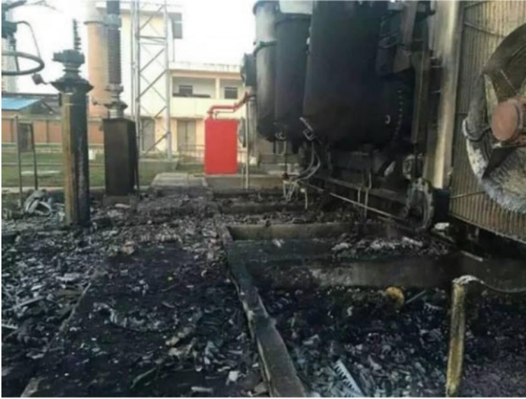
Fig. 3.1 Internal damage scene of power facilities
