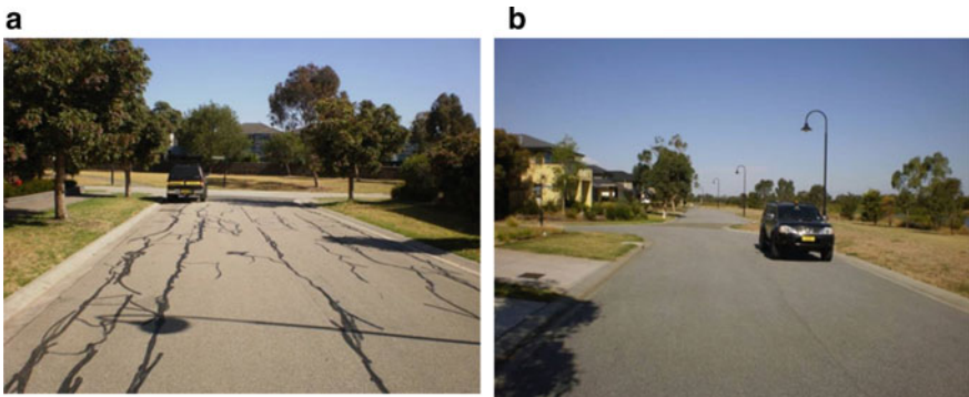
Fig. 9 a Cracked seal: base not stabilized. b Good seal: enzyme-stabilized base
