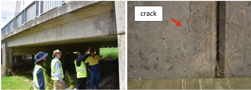
Fig. 2 A 25-year-old bridge in New South Wales, Australia, suffering from alkali-silica reaction
