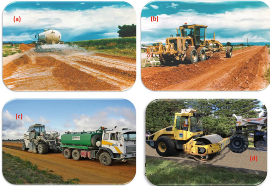
Fig. 4 a For an optimum moisture content mix water lightly through the broken soil. b Ripping and shaping an existing road base. c Adding stabilizer using a mixing machine and water tanker in tandem. d Compaction by 16-tonne vibrating roller
