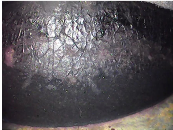
Fig. 4 Appearance detection image 2 of rubber bearing
