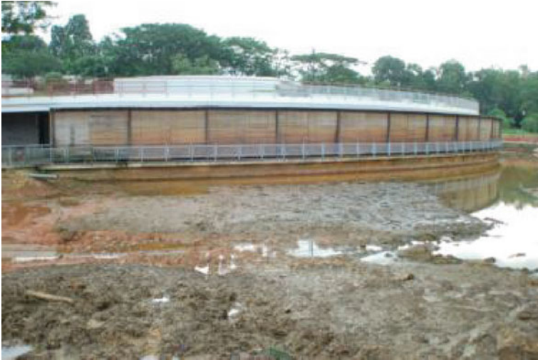
A sedimentation basin with sediment collected.
