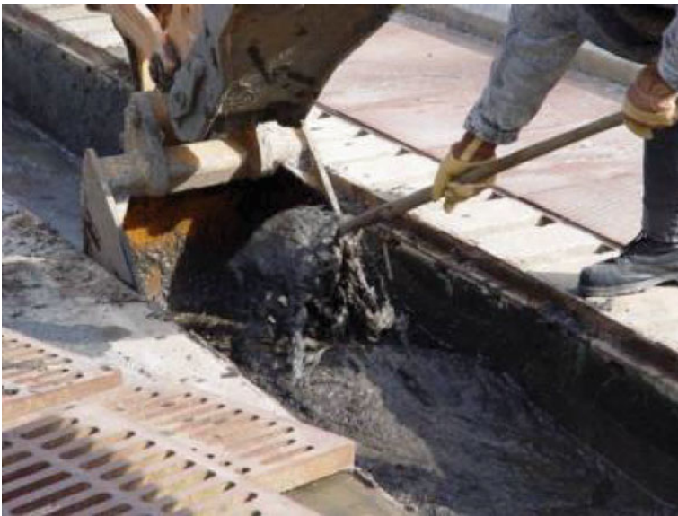
Shoveling accumulated gross solids and sediment into the bucket of a backhoe.
