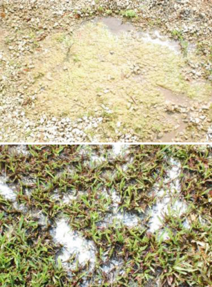
Moss, other vegetation and water at the surface of an infiltration trench are signs that the practice is clogged and not infiltrating.
