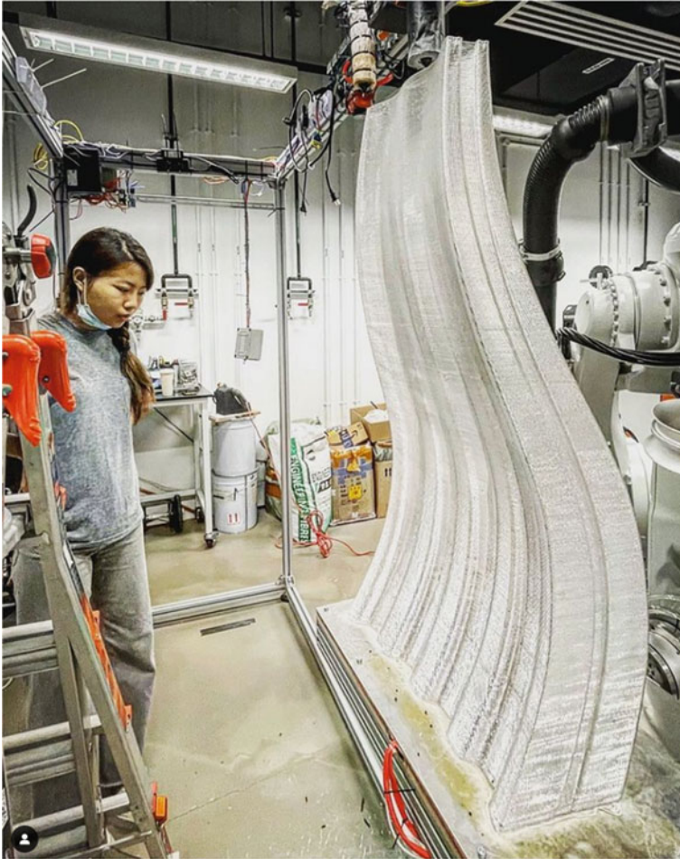
Fig. 5. Printing process for a large piece of the dome. The 1.5 m tall piece is almost complete. The Robot positions a heated built plate (bottom of the image), while the extruder is stationary on a frame (top of the image).
