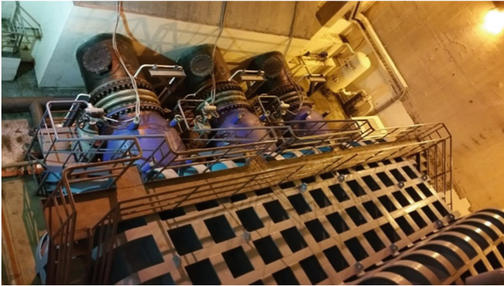
Fig. 8. Filling valves of F/E system
