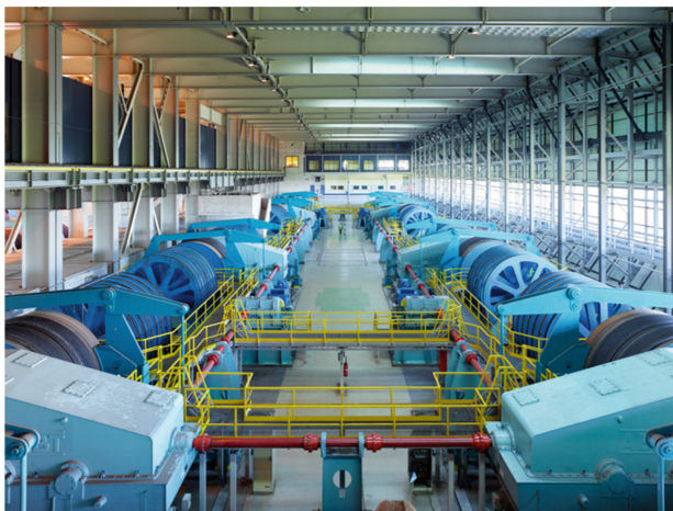
Fig. 3. Machine hall of Strépy-Thieu Shiplift
