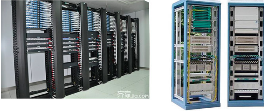
Fig. 2.8 Cable distribution cabinet in common use
