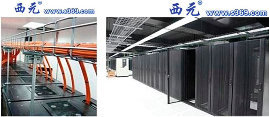
Fig. 2.67 Ceiling-mounted cabling channels
