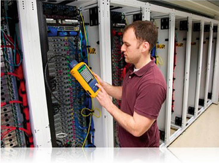
Fig. 2.51 Troubleshooting using a network tester
