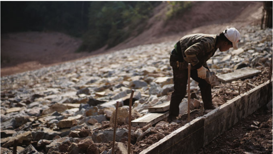
Fig. 3 A worker constructs a Vietnamese-funded irrigation dam within Nam Ha National Protected Area. Photo by Brian Cheang (March, 2019)
