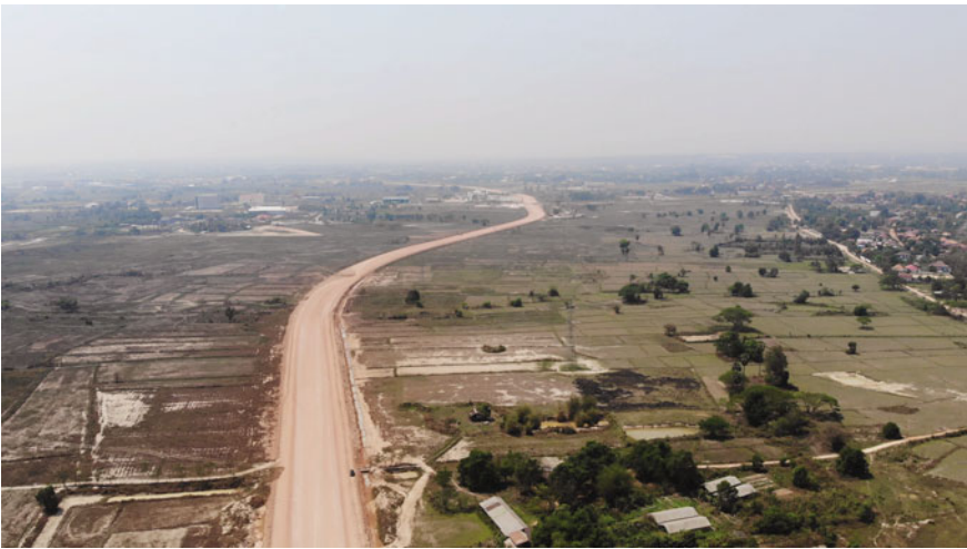
Fig. 4 A highway, crossing largely disused farmland, under construction in Vientiane linking the capital's airport to a planned station on the China-Laos Railway. Panyanivej Organic Farm, a social enterprise formerly part of the Participatory Development Training Centre (PADETC), Laos's oldest but politically accosted civil society organization focused on sustainable development, is bisected by the highway yet continues operation. Photo by Xiaoxuan Lu (March, 2019)
