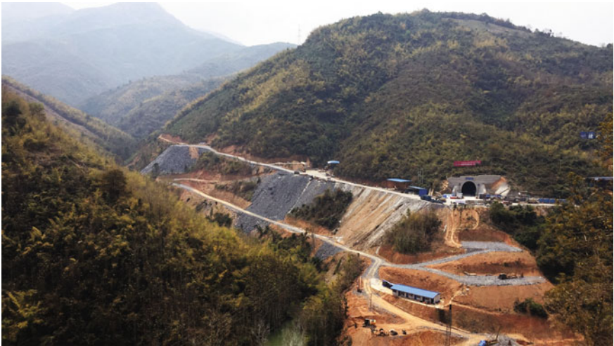
Fig. 2 A tunnel portal of the China-Laos Railway under construction above the Nam Khan River south of Luang Prabang. Photo by Ashley Scott Kelly (March, 2018)
