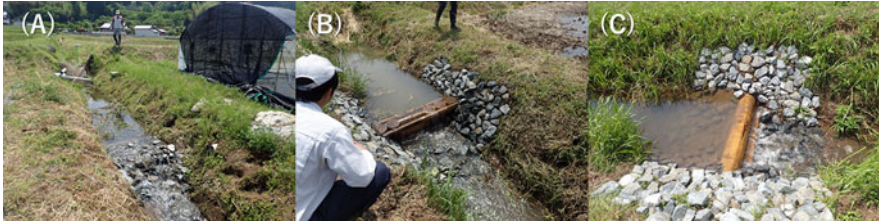
Fig. 12.5 Resulting structure of dams. Dams create permanent aquatic areas and step-pool structures in the channels. Dams were built using three types of materials. (a) Stonework. (b) Flashboard. (c) Log
